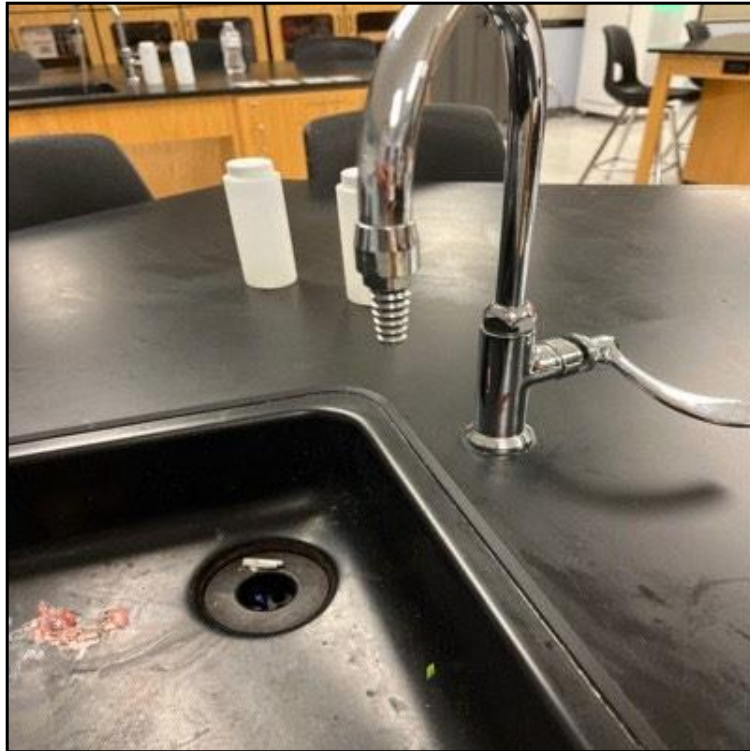
View of potential DWO and sample 04-01-105-CF-P-15 (No sample taken. Outlet was offline.)
