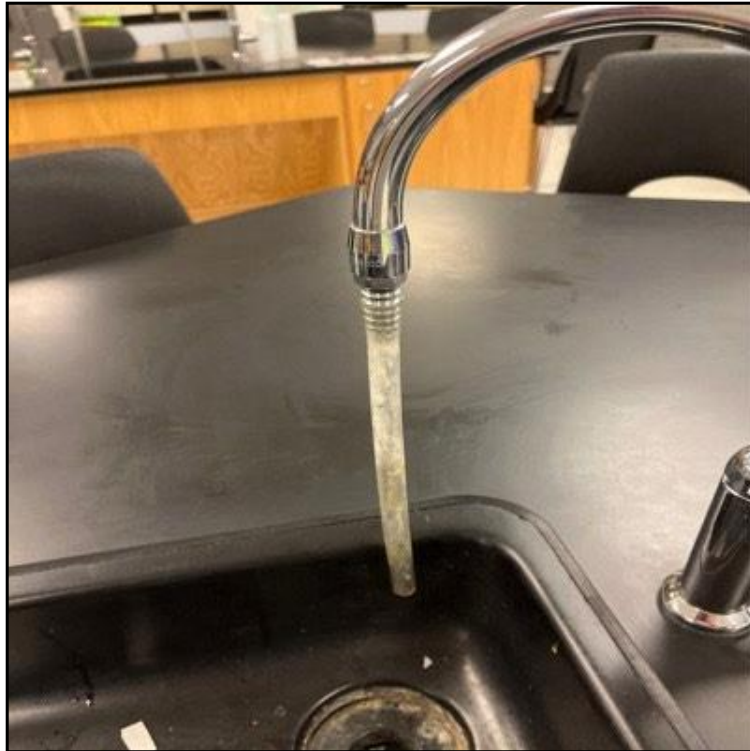
View of potential DWO and sample 04-01-105-CF-P-17 (No sample taken. Outlet was offline.)
