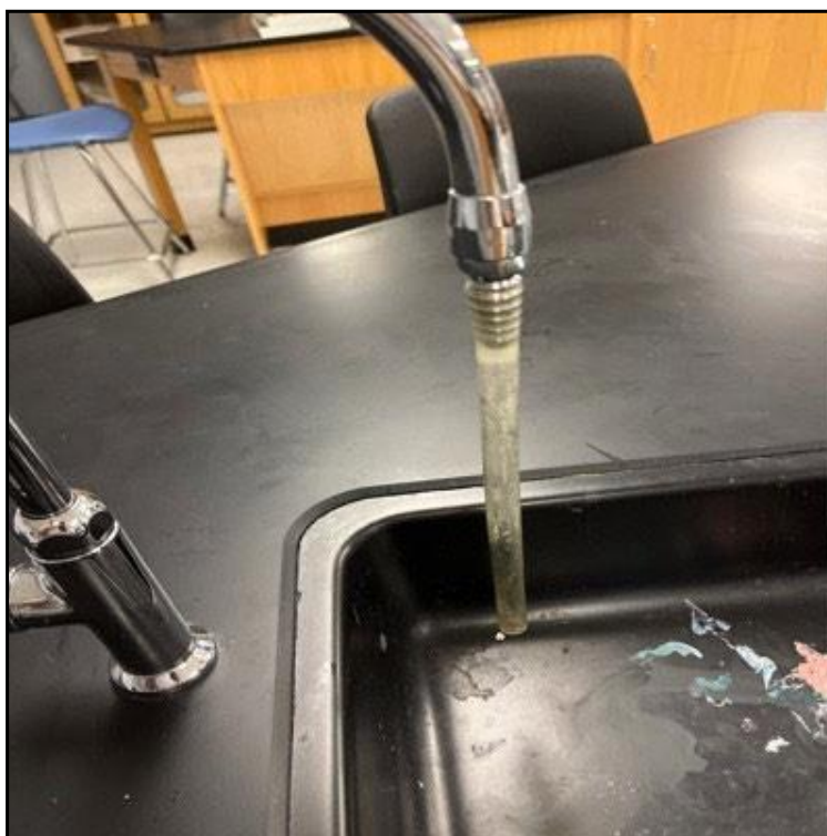
View of potential DWO and sample 04-01-105-CF-P-14 (No sample taken. Outlet was offline.)
