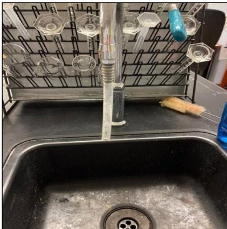
View of potential DWO and sample 04-01-105-CF-P-13 (No sample taken. Outlet was offline.)
